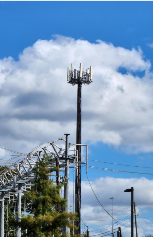
Communications tower near Crown Castle HW in Houston.
